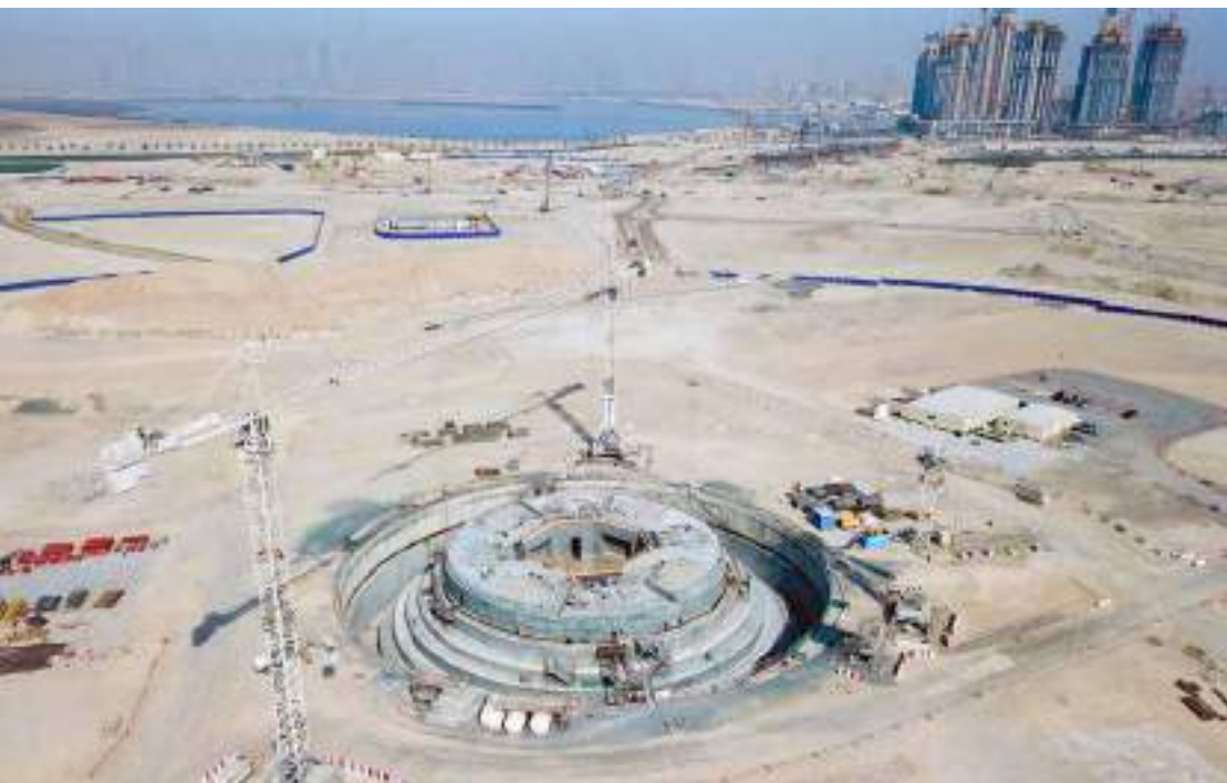
CLOCKWISE FROM LEFT: FOUNDATIONS FOR THE TOWER AT DUBAI CREEK HARBOUR, SWRO DESALINATION PLANT AT JEBEL ALI POWER STATION, WARNER BROS. WORLD ABU DHABI
